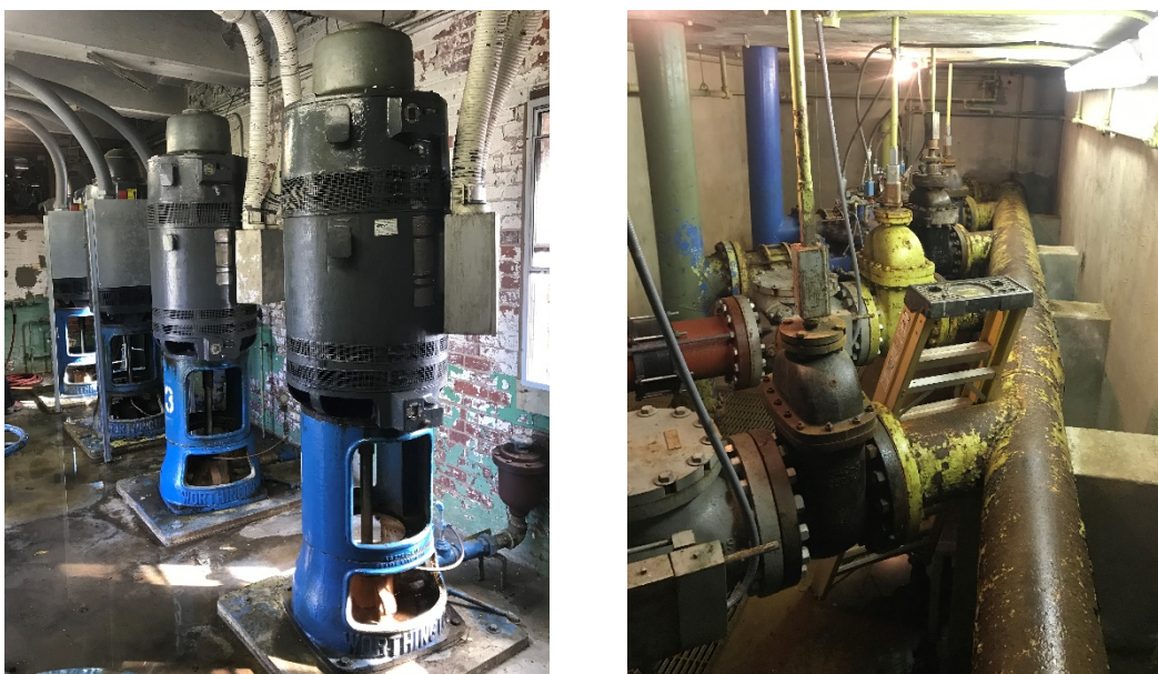
Figure 5.5: Existing Vertical Turbine Pumps and Discharge Piping
