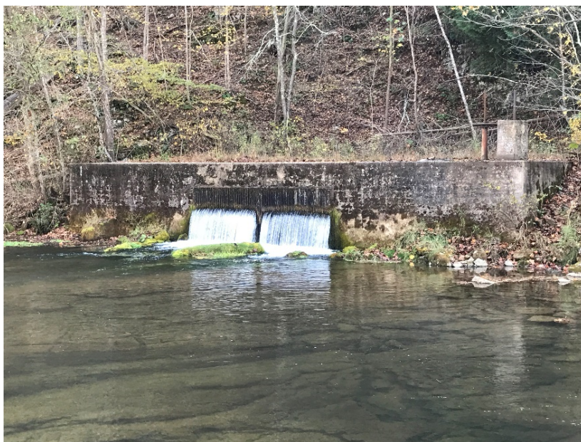
Figure 2.8: Gardner Spring Box adjacent to the Middle River
