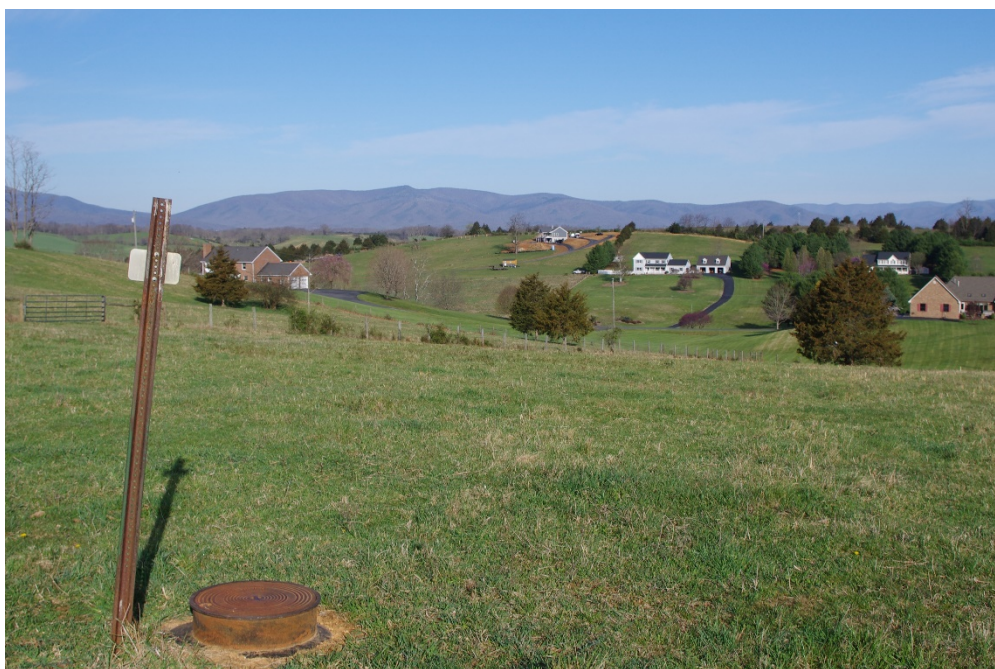
Figure 6.2: Air Relief Valve Along Water Line Route
