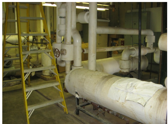
Piping in Laundry
