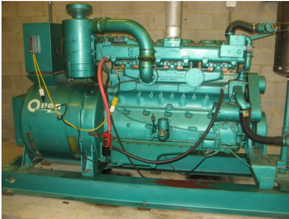
Emergency Generator at Building 122
