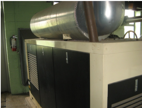
Standby Generator in Power Plant
