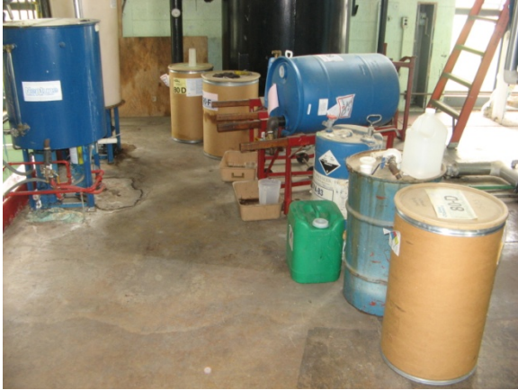
Water Treatment Chemicals in Power Plant
