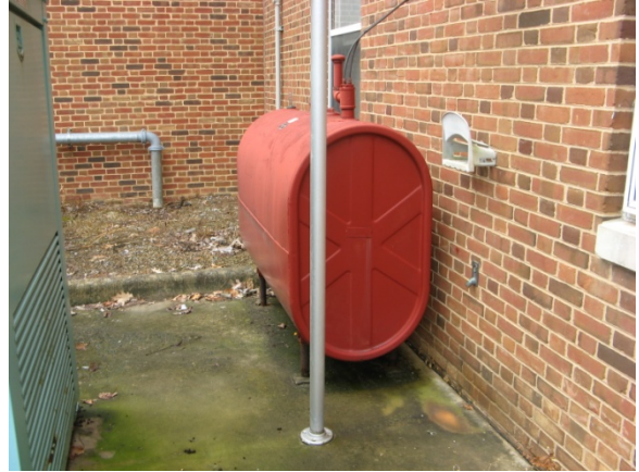
AST at Building 107
