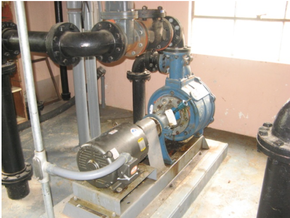
Wastewater Pump in WWTP Pump Station
