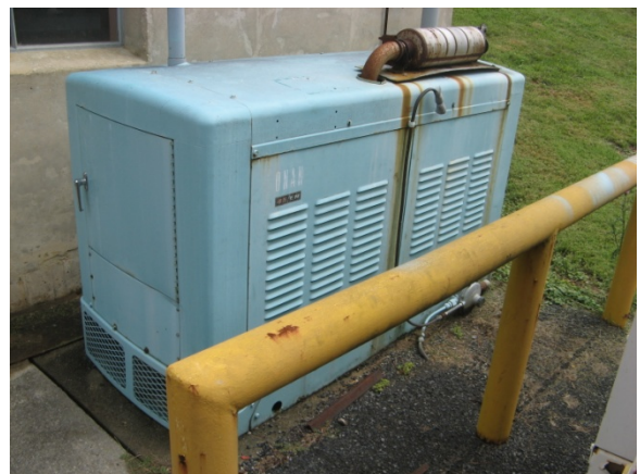
Emergency Generator at WWTP Pump Station
