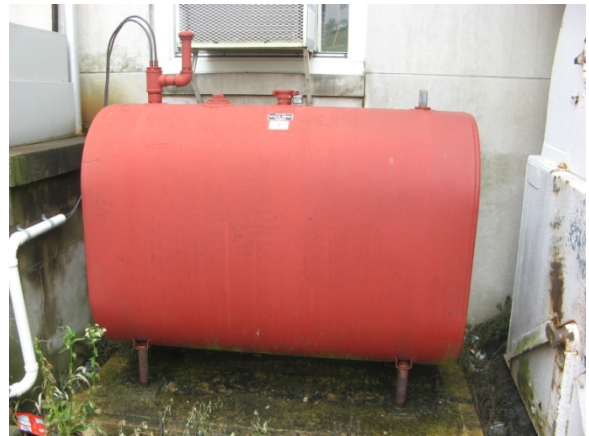
AST at Building 103
