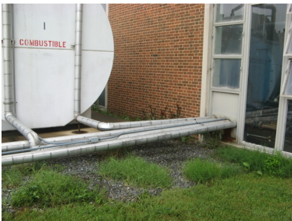
Fuel Feed into Power Plant
