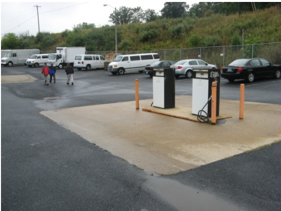
Fuel Pumps at Physical Plant Services/Materials Management Building
