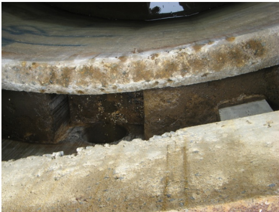
Emergency Overflow Tank at WWTP Pump Station
