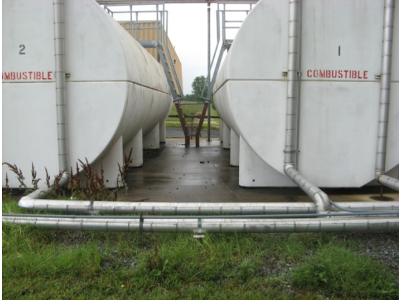
ASTs at Power Plant
