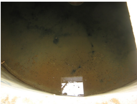
Emergency Overflow at WWTP Pump Station
