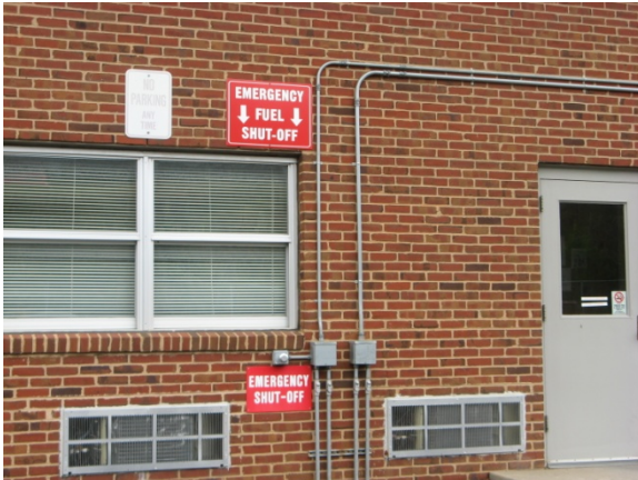
Emergency Fuel Shutoff at Physical Plant Services/Materials Management Building
