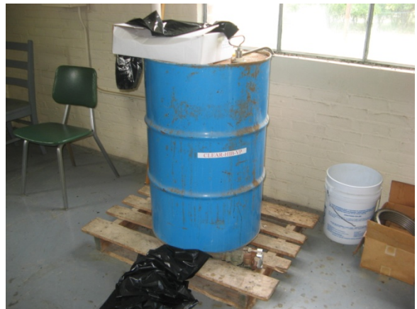
Water Treatment Chemical Storage in WWTP Pump Station
