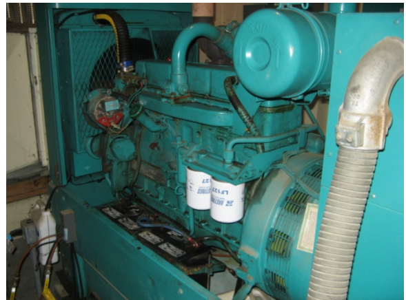
Emergency Generator at Building 127
