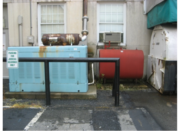
AST at Building 103
