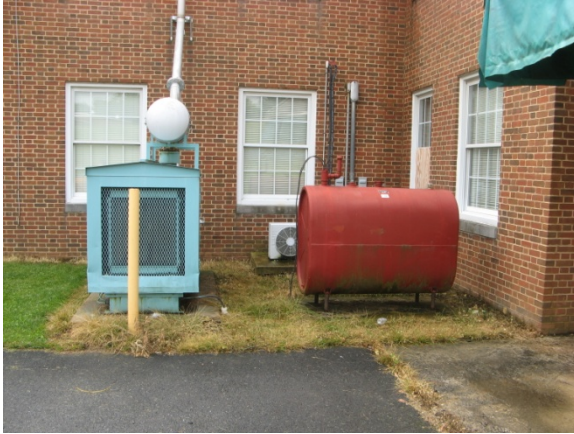
AST at Building 115
