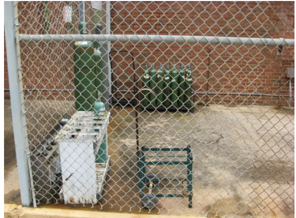
Oxygen Storage at Building 122
