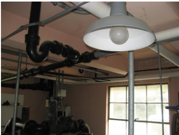
Interior of WWTP Pump Station
