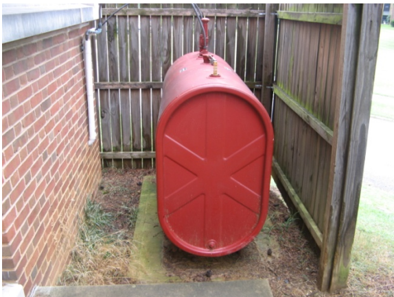
AST at Building 122
