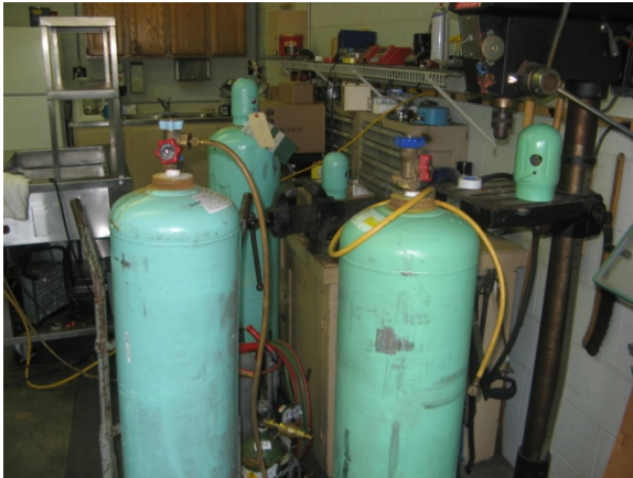
Freon Cylinders in Physical Plant Services/Materials Management Building
