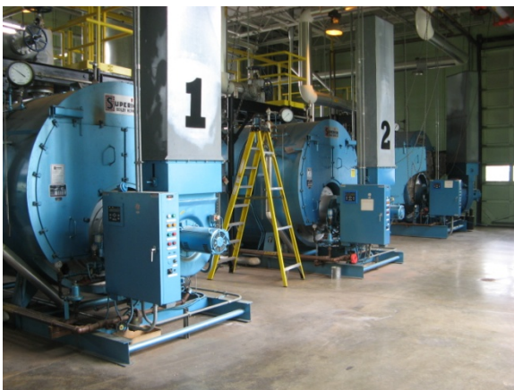
Boilers in Power Plant
