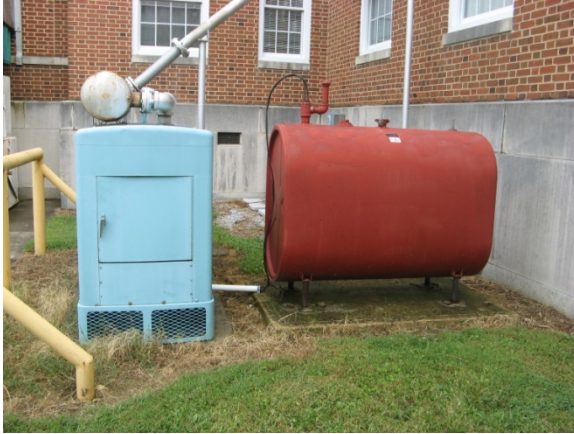
Generator and AST at Building 102
