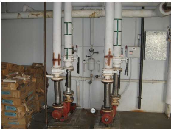
Piping in Mechanical Room of Physical Plant Services/Materials Management Building
