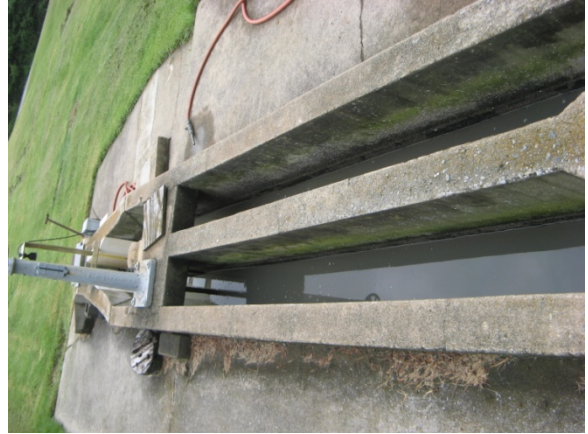
Wastewater Influent Flow Channel
