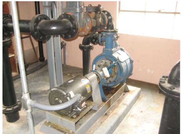
Wastewater Pump in WWTP Pump Station
