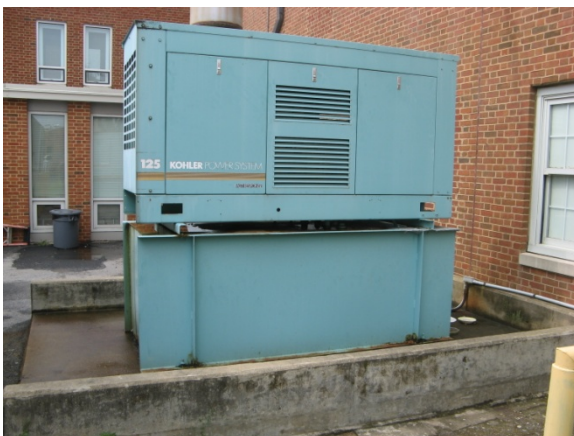
Generator and AST at Building 118
