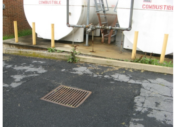
Fill Port of ASTs at Power Plant
