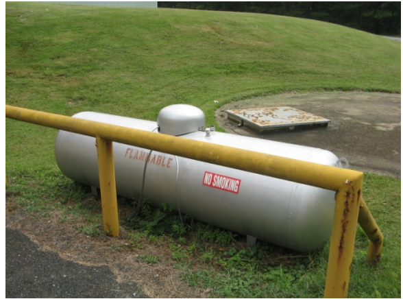
Propane Tank at Emergency Generator at WWTP Pump Station
