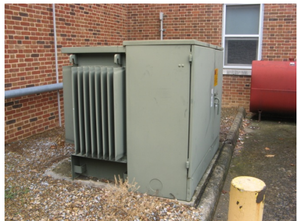
Transformer at Building 107
