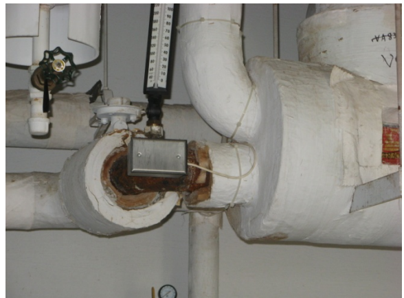
Pipe Insulation in Physical Plant Services/Materials Management Building
