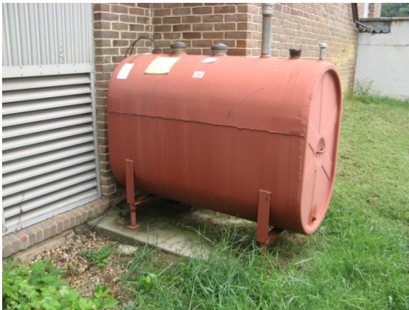
AST at Building 127
