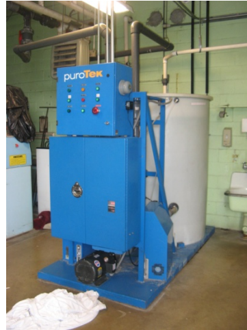
Water Treatment System in Laundry
