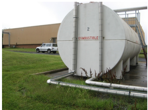
Fuel Feed into Power Plant
