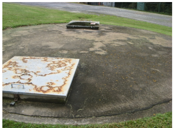
Emergency Overflow at WWTP Pump Station
