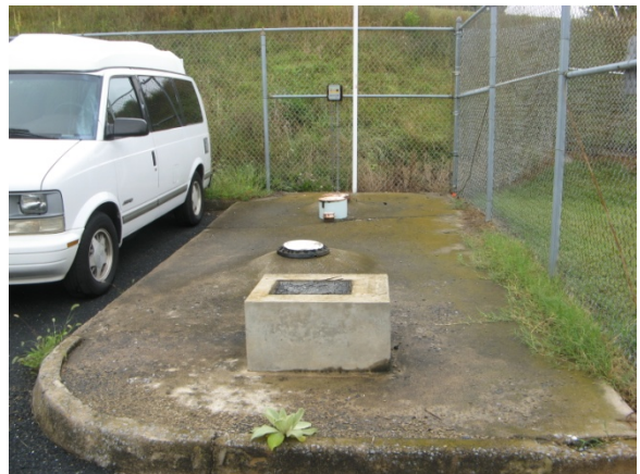
Fill Ports for USTs at Physical Plant Services/Materials Management Building
