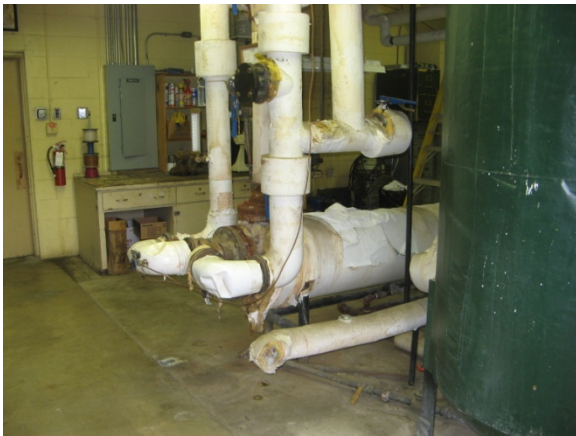
Piping in Laundry
