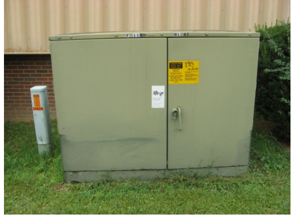
Transformer Outside of Laundry
