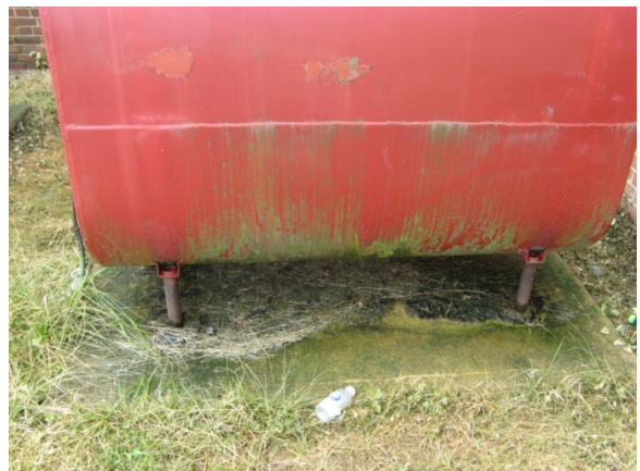
AST at Building 115
