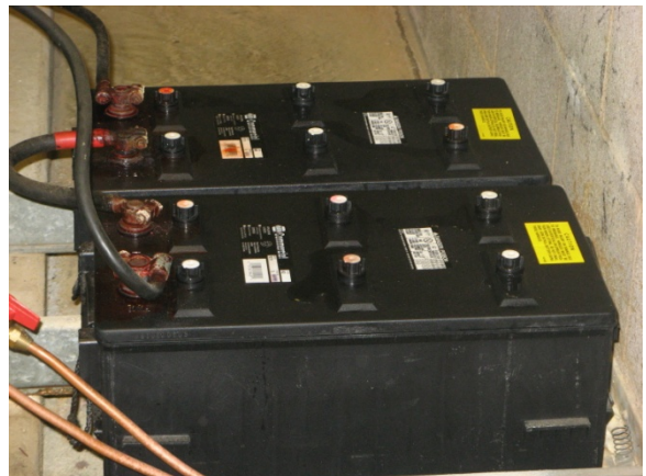
Batteries for Emergency Generator in Building 122
