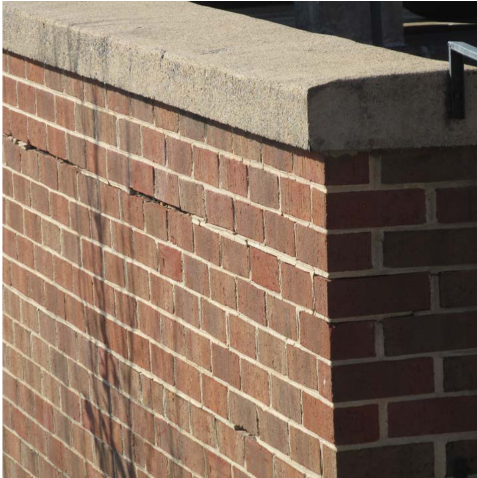
Photo 21 - View of the exterior face of the masonry wall along the east side of the parking garage. We noted cracked and loose or missing mortar in the joints in the brick veneer.
