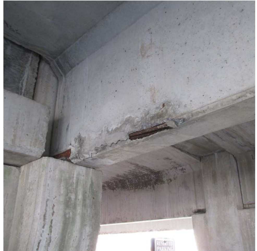
Photo 2 - View of the bearing end of a precast concrete single tee. We noted that a previous repair in the vicinity of the end of the tee had spalled partially exposing the steel reinforcement.
