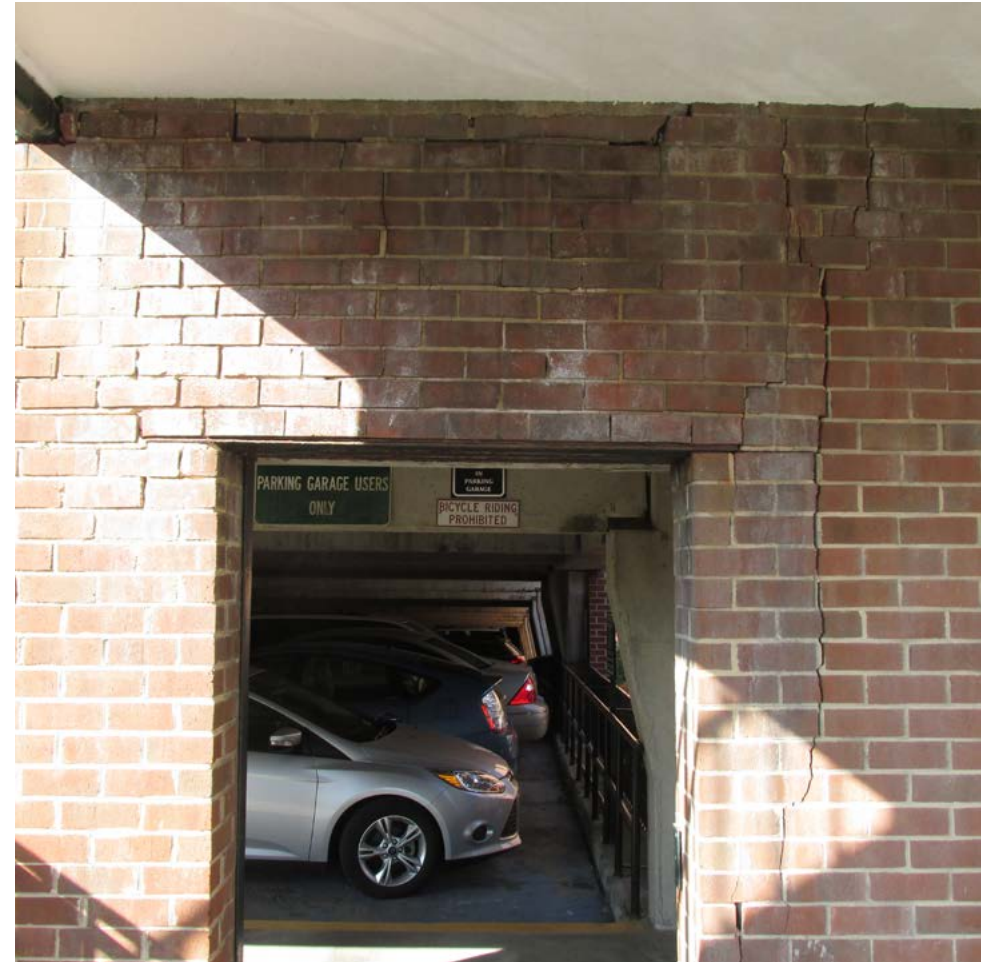
Photo 22 - View of the entrance to the 2B level of the parking garage at the northeast corner of the parking garage. We noted vertical, horizontal, and stairstep cracks in the brick and mortar joints of the masonry wall. We also noted loose and or missing mortar in the joints of the brick veneer. Additionally, we noted the steel angles forming the lintel above the opening were rusted.
