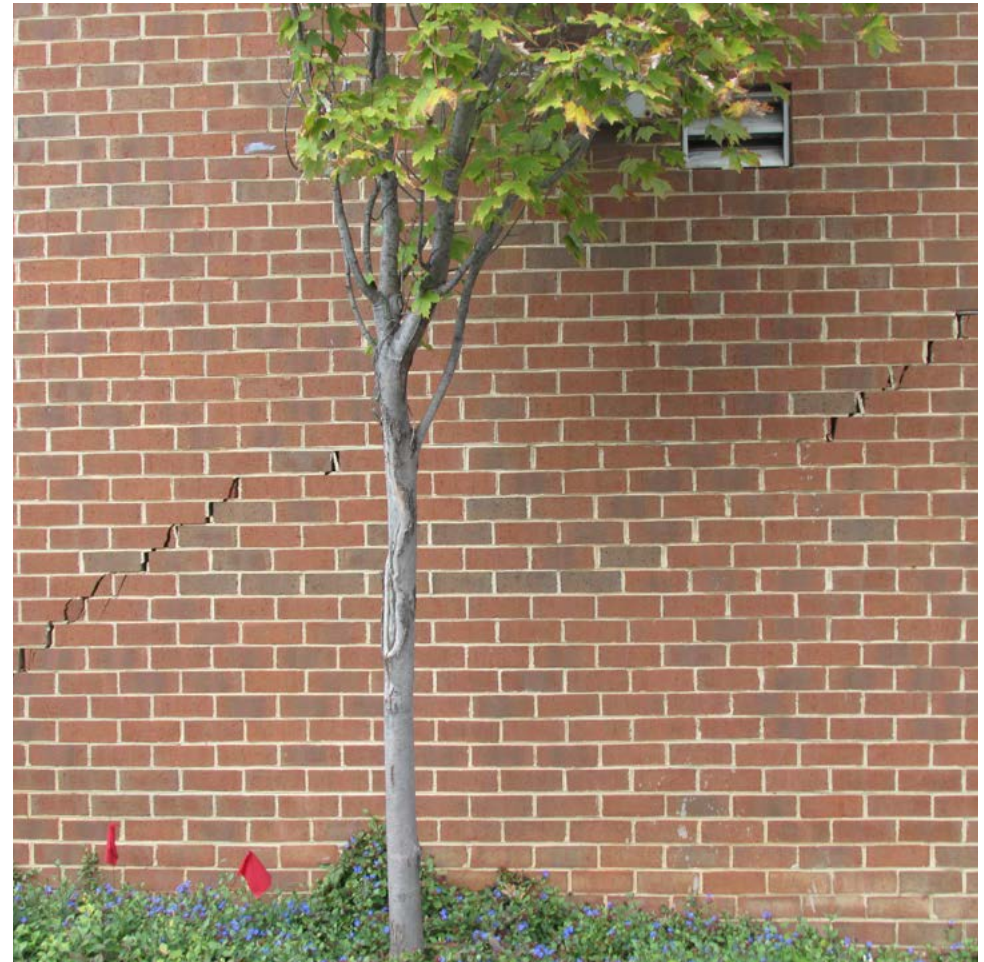
Photo 26 - View of the exterior face of the masonry wall to the west of the main entrance to the parking garage off of Johnson Street. We noted the presence of horizontal and stairstep cracks in the bricks and mortar joints of the brick veneer. The cracks were a maximum of approximately 3/4" wide at some locations.
