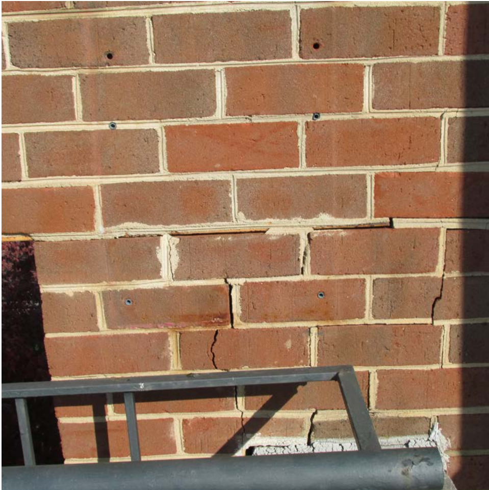
Photo 23 - Close-up view of the brick veneer at the top level of the elevator shaft. This photo was taking looking towards the north. We noted that a portion of masonry wall overhangs the lower section of the wall and is supported by a steel plate that is embedded approximately 24" into the wall. We noted horizontal and stairstep cracks in the brick and mortar joints of the brick veneer at this location.
