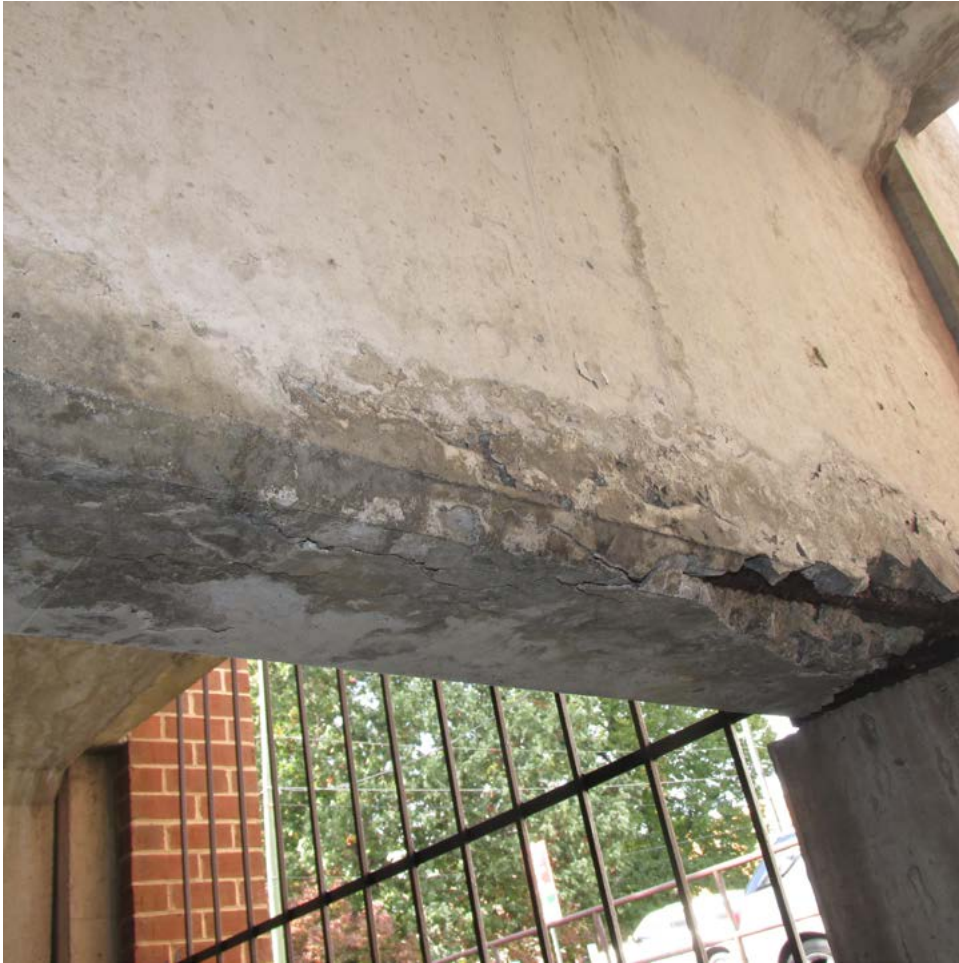
Photo 7 - Close-up view of the bearing end of a precast concrete single tee. We noted that the bearing end of the tee had been previously repaired and that cracking and spalling of the repair had partially exposed the reinforcement.
