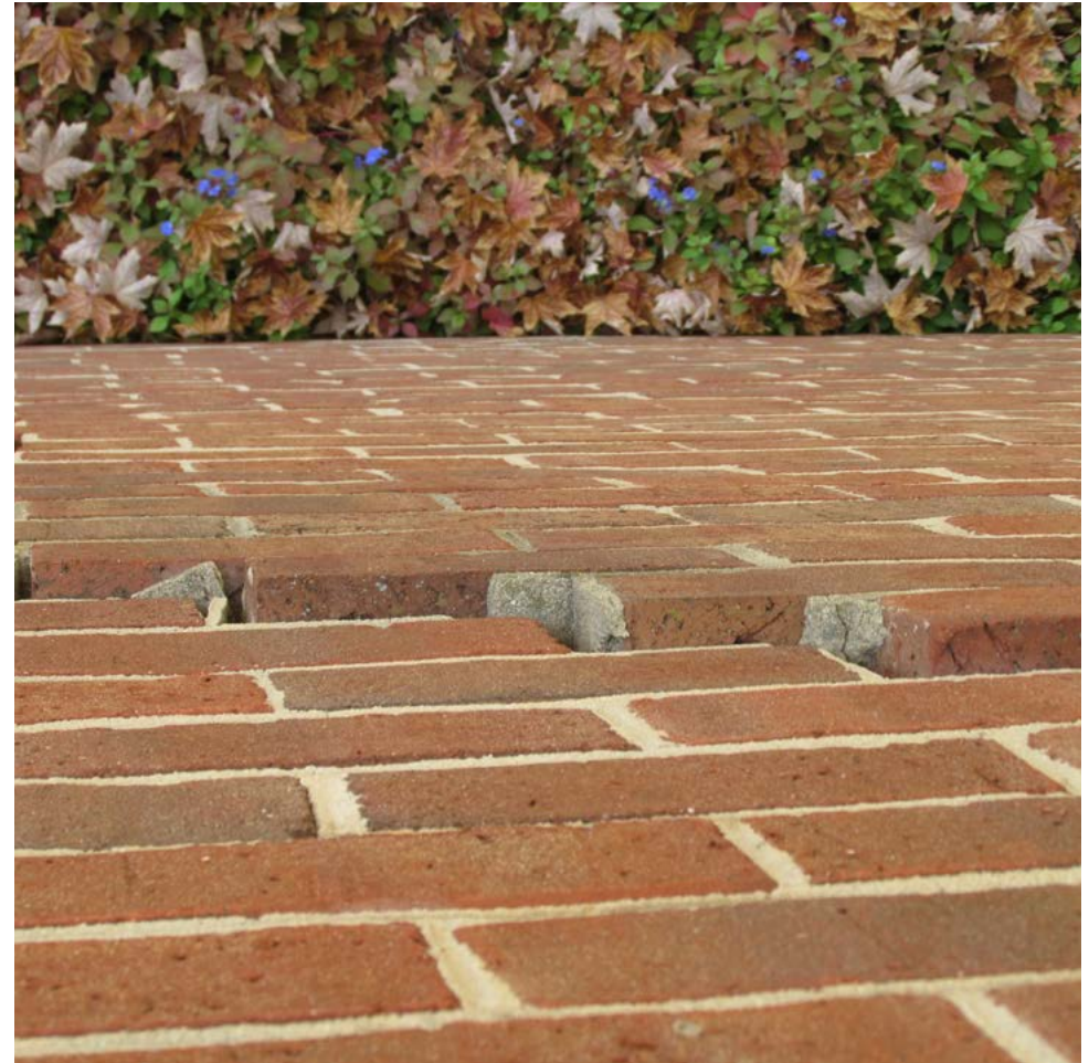
Photo 24 - View looking down the exterior face of the masonry wall located below the pedestrian ramp leading to South Lewis Street at the northwest corner of the parking garage. We noted the presence of stairstep and vertical cracks in the bricks and mortar joints of the brick veneer. Additionally, we noted that the bricks above the crack were displaced from those below the crack.
