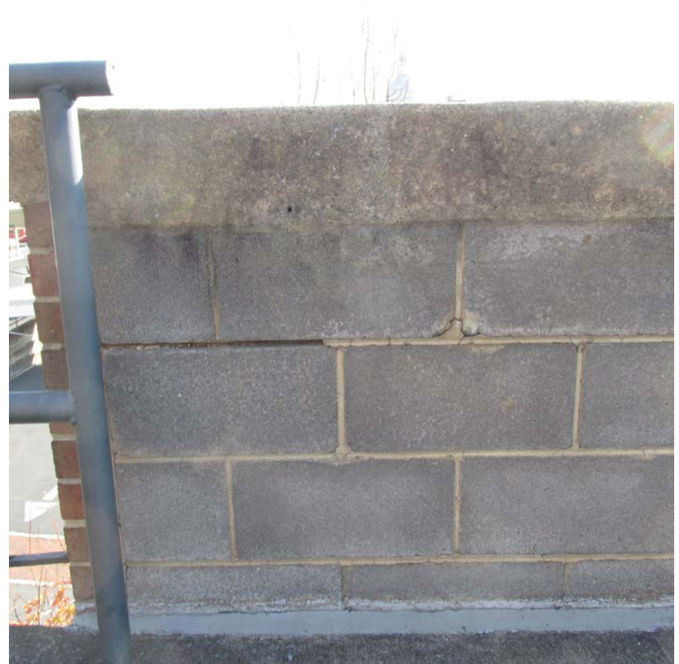
Photo 20 - View of the interior face of the top of the masonry wall at the east side of the parking garage. We noted horizontal cracks in the mortar joints. Additionally, we also noted missing and loose mortar.
