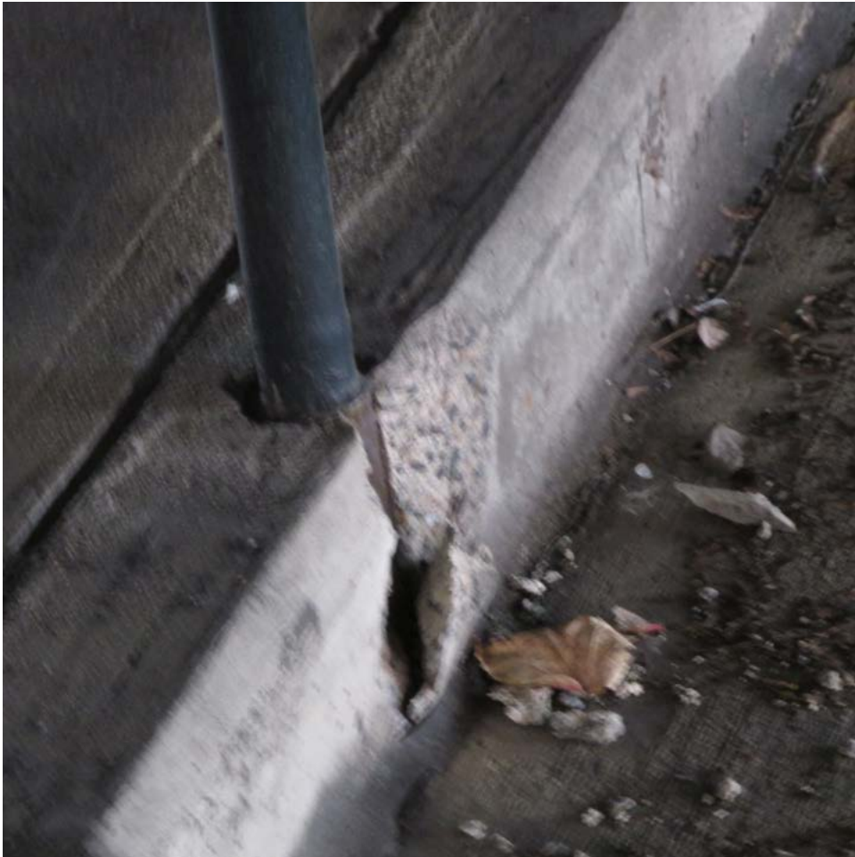
Photo 15 - Close-up view of a steel guardrail post embedded in the cast-in-place concrete curb separating two levels of the parking garage. We noted the face of the concrete curb had spalled at the location of the sleeve embedded into the concrete for the guardrail post.
