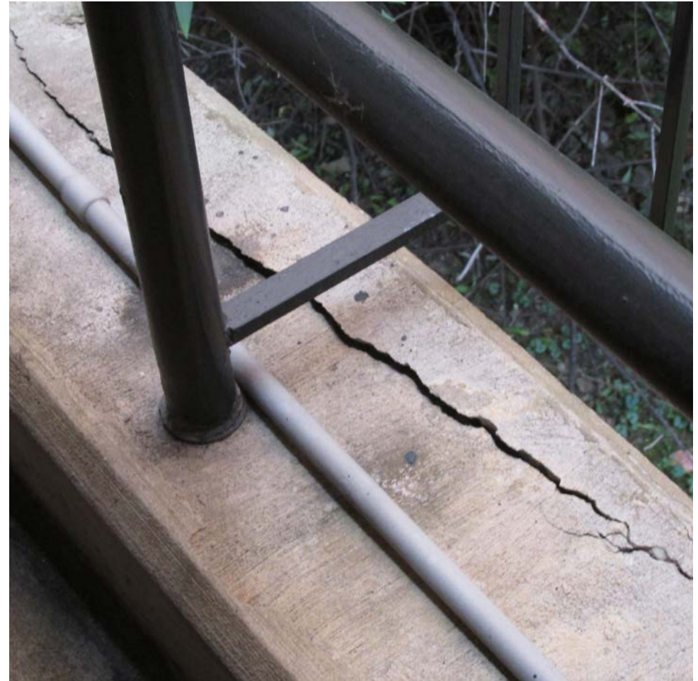
Photo 16 - Close-up view of the cast-in-place concrete edge beam along the north side of the parking garage. We noted that the concrete beam was cracked and spalled along this section of the parking garage.
