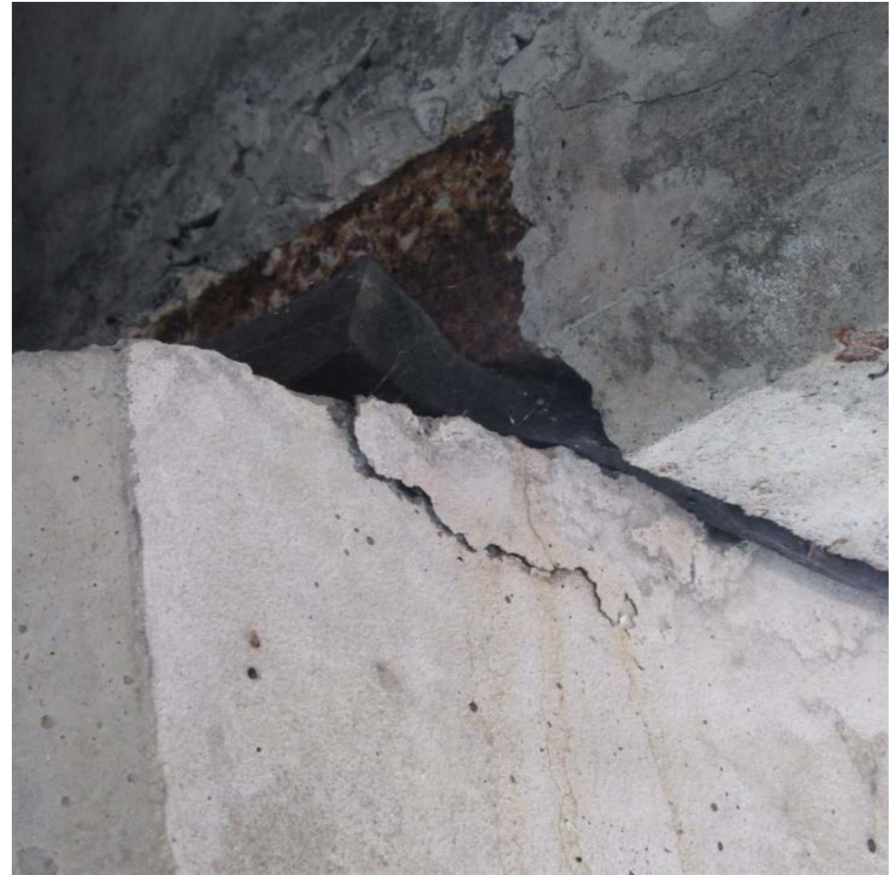
Photo 4 - Close-up view of the bearing of a precast concrete single tee on a precast concrete column. We noted that the bearing pad was flattened and deformed. We also noted a spall in the precast concrete column at the edge of the bearing.
