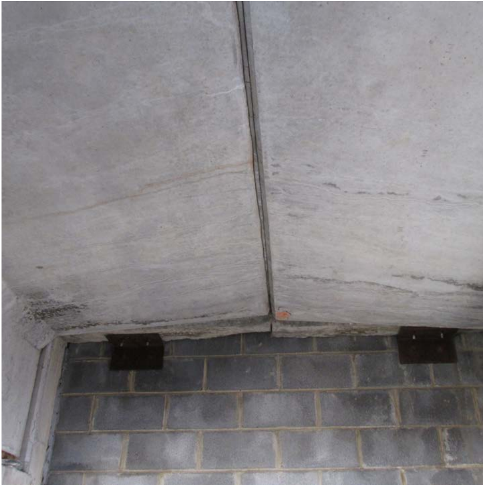
Photo 1 - View of the underside of two adjacent precast concrete single tees at the upper level of the parking garage. This photo was taken looking towards the south end of the parking garage. The flanges of the single tees were vertically offset approximately 1 1/2 inches from each other. We also noted a spall in the precast concrete at the corner of the rightmost panel near the edge.
