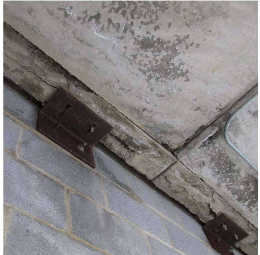
Photo 18 - View of the underside of the cast-in-place concrete beam along the south side of the parking garage. We noted cracking and spalling of the concrete which partially exposed the steel reinforcement. Additionally, several rusted steel brackets anchoring the wall to the cast-in-place concrete beam were observed. Loose and or missing anchor rods and nuts were observed at several of the holes in the steel brackets.
