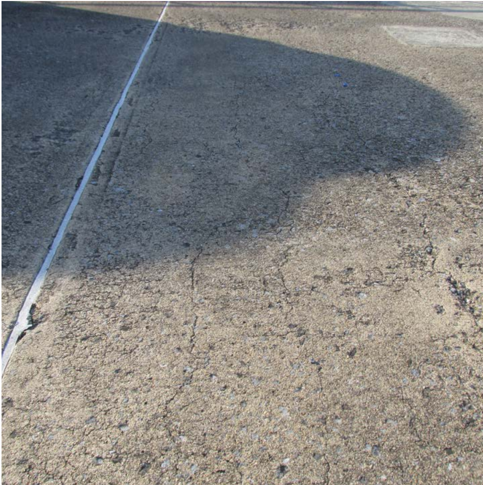
Photo 11 - View of the topping slab of the parking garage at the upper level of the garage. The topping slab showed signs of loss of cement paste at the surface partially exposing the aggregate. Several cracks and spalls were present in the topping slab.
