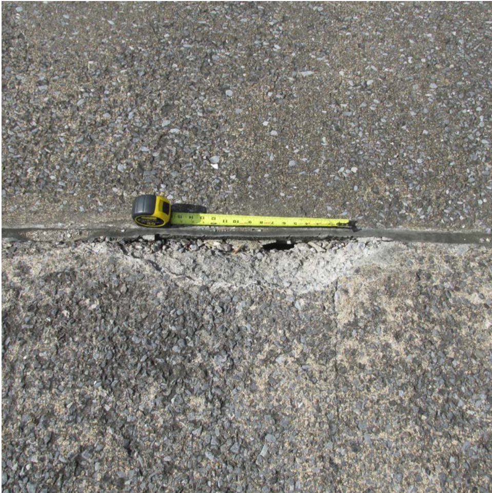
Photo 13 - Close-up view of the joint in the topping slabs between two adjacent precast concrete single tee planks. We noted a spall that extended the full depth of the topping slab exposing a gap between the adjacent single tee planks.
