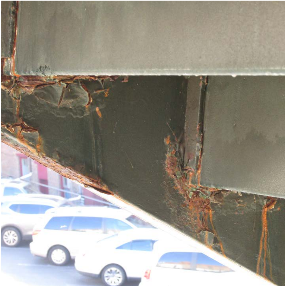
Photo 27 - Close-up of the underside of the steel stair stringers of the exterior stair along the east side of the parking garage. We noted that the metal stair pans were supported by steel bars welded to the stair stringer. Corrosion of the stringer, support bars, and metal stair pans were observed.
