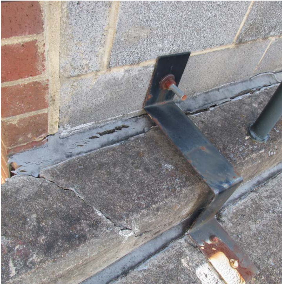
Photo 19 - Close-up view of bent steel strap anchor bolted into the masonry wall at the southeast corner of the parking garage at the upper level. Note the large caulk joint between the wall and the cast-in-place concrete curb. Additionally we noted a crack in the cast-in-place concrete curb adjacent to the end of the masonry wall.
