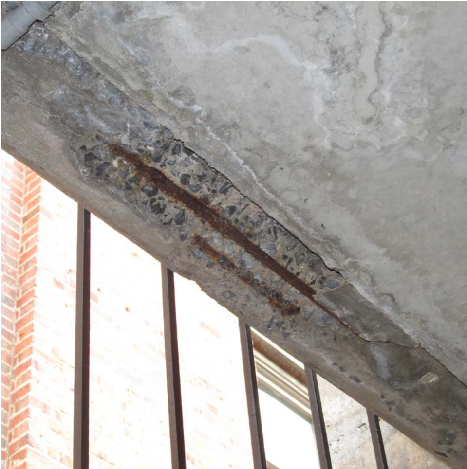
Photo 17 - View of the underside of the cast-in-place concrete beam along the north side of the parking garage. We noted spalling of the concrete which partially exposed the steel reinforcement. Additionally, the exposed steel reinforcement showed signs of corrosion.
