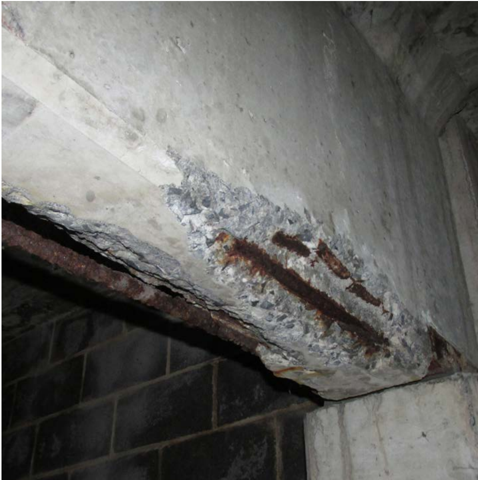
Photo 9 - Close-up view of the bearing end of a precast concrete single tee. We noted spalled concrete exposing the steel reinforcement at the bearing end of the tee. We also noted that the exposed steel reinforcement showed signs of corrosion.
