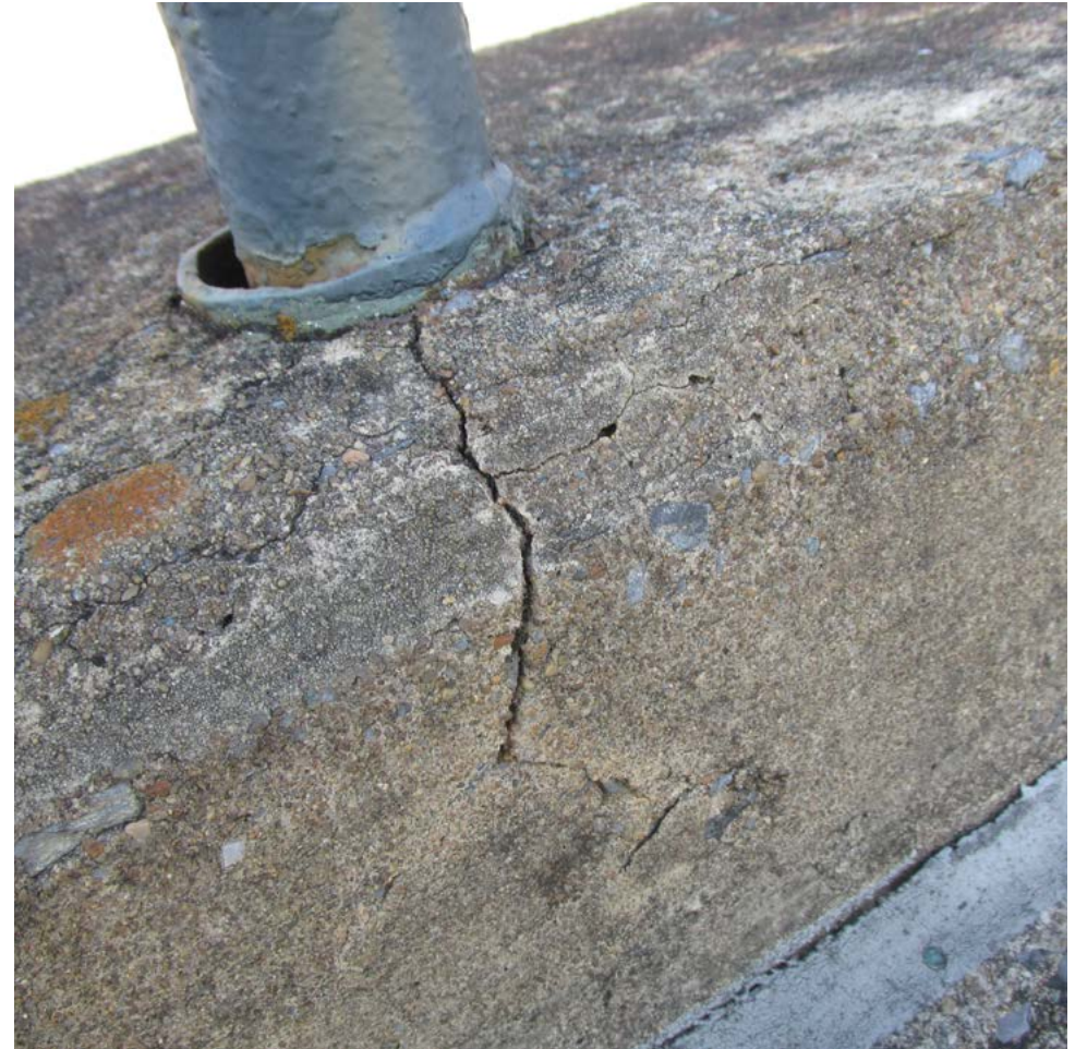
Photo 14 - Close-up view of a steel guardrail post embedded in the cast-in-place concrete curb separating two levels of the parking garage. We noted a vertical crack extending out from the embedded guardrail and continuing down both sides of the cast-in-place concrete curb.
