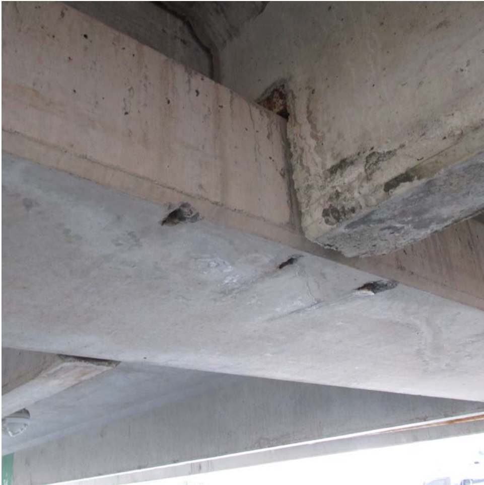
Photo 3 - View of a precast concrete beam spanning above the drive lane at the east end of the parking garage. We noted the presence of several spalls in the precast concrete beam which partially exposed the steel reinforcing.
