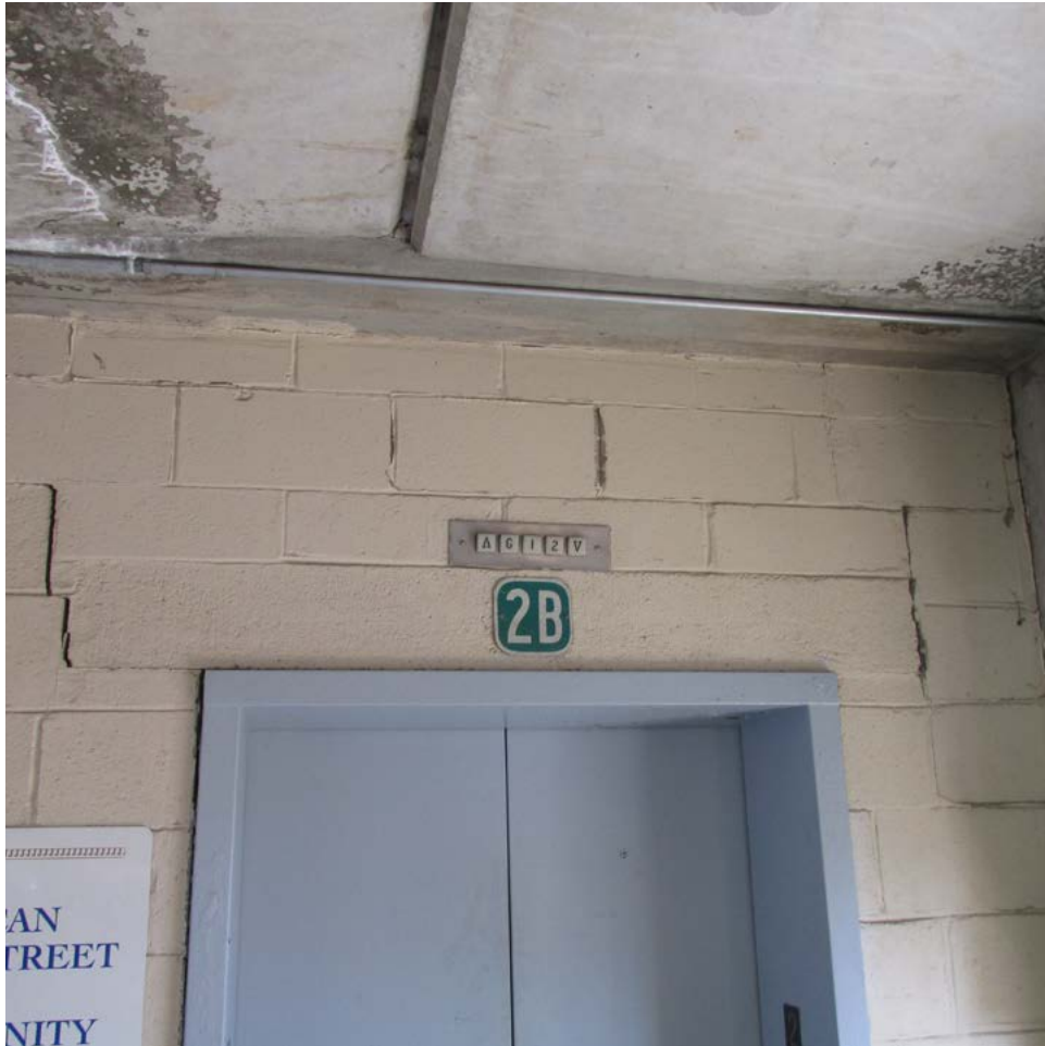
Photo 25 - View of the interior face of the masonry wall for the elevator enclosure at level 2B. The photo is taken looking towards the north. We noted stairstep and horizontal cracks in the mortar joints of the CMU wall. Additionally, the flanges of the interior and end single tee precast concrete planks were vertically offset approximately 1 inch from each other.
