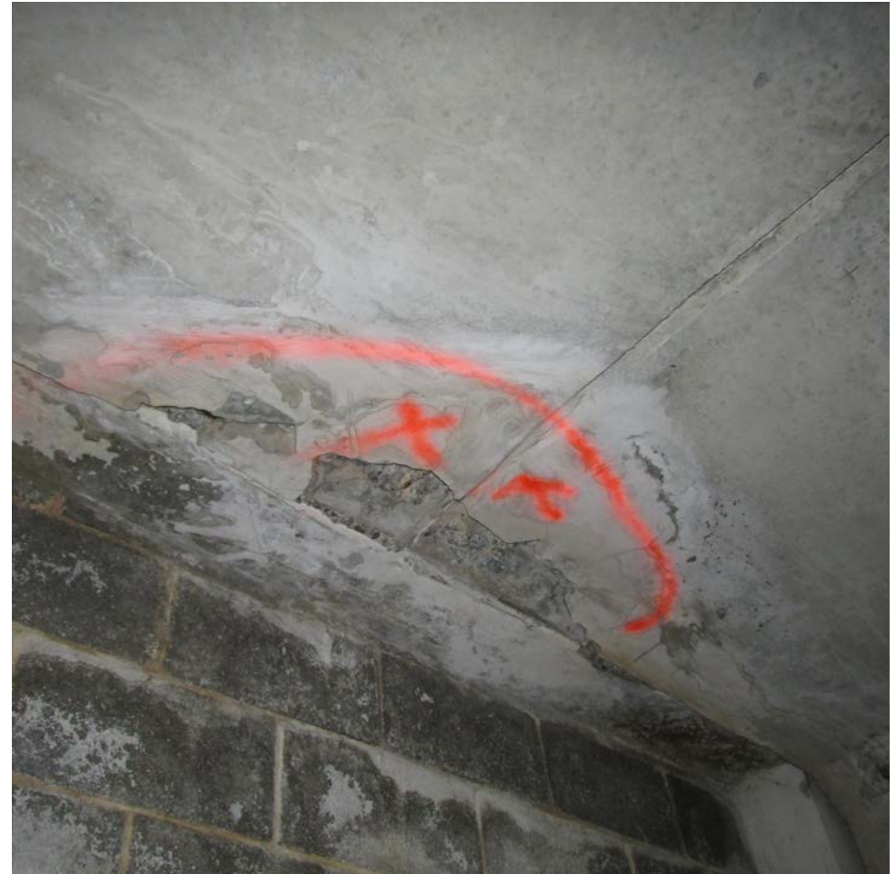
Photo 10 - View of the underside of two precast concrete single tees. We noted spalling of the concrete which partially exposed the steel reinforcement at the end of the two tees.
