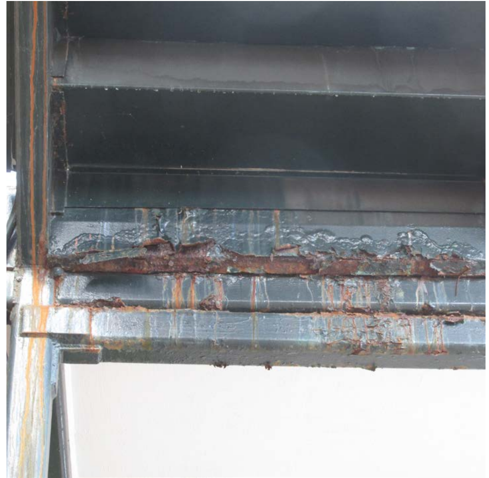
Photo 28 - View of the underside of the exterior steel stair along the east elevation of the parking garage. We noted corrosion of the metal stair pan and supporting steel framing.
