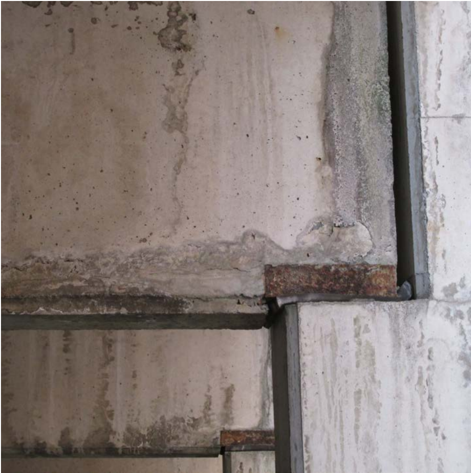
Photo 5 - Close-up view of the bearing end of a precast concrete single tee. We noted that the bearing end of the tee had been previously repaired and that new cracks have formed along the edge of the repair.
