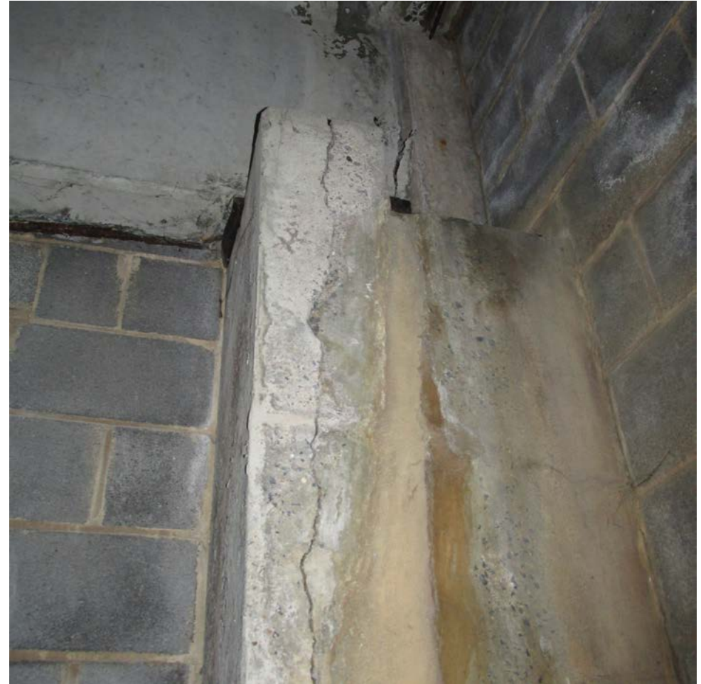
Photo 8 - View of the precast column at the north end of the parking garage. We noted the presence of a vertical crack in the precast concrete column extending down from the bearing end of the precast concrete single tee. We also noted a spall on the far side of the precast concrete single tee which partially exposed the steel reinforcement at the bearing end.
