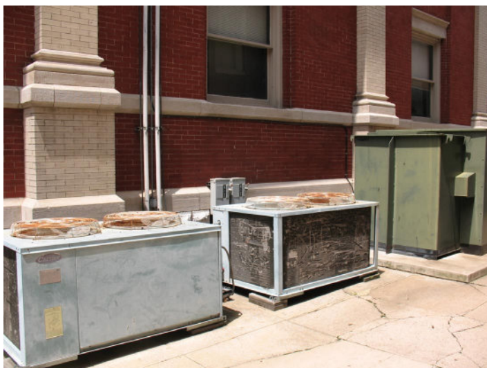
Mechanical units and transformer located on the east side of the building.
