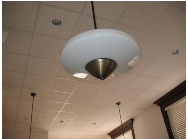
Non-original Art-Deco style fixtures seen in several spaces throughout the building.
