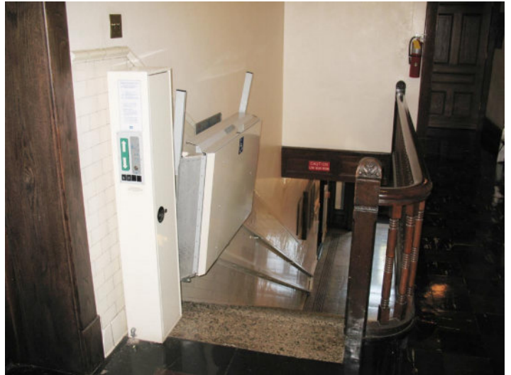
Handicap stair lift used to bring wheelchairs to the second floor.
