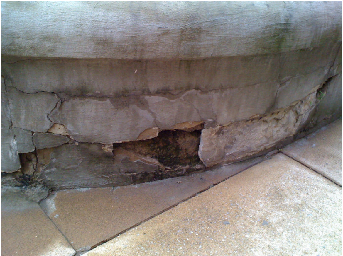
Photo #12: Severe spall at base of landing wall
