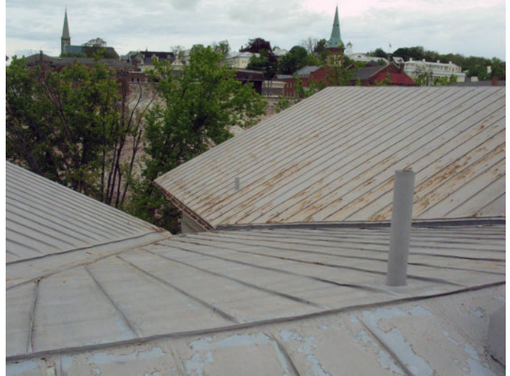
View of roof of the addition showing rusted roof areas. Also, note half-round gutter.
