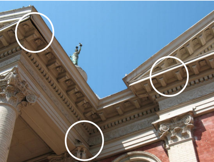
Detail of sheet metal cornice with circled areas showing typical deterioration and missing elements.
