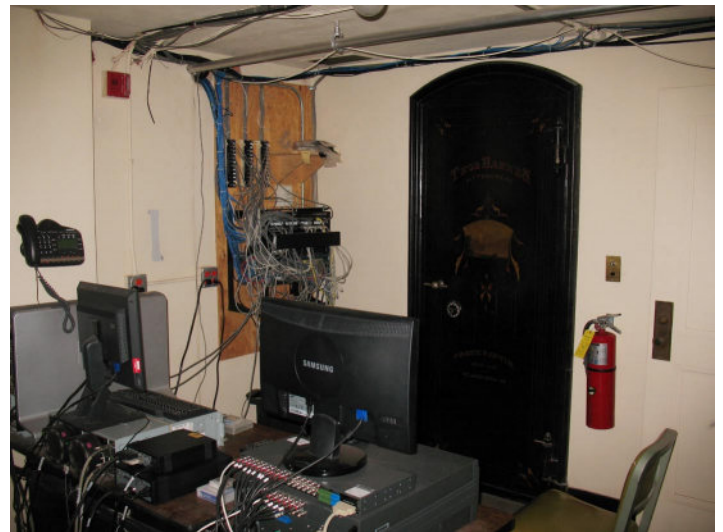
Evidence vault and server equipment located in the basement. The door of the vault was reused from the previous courthouse.
