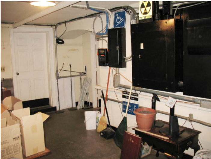
Electrical service and panels in the basement are outdated and would be upgraded in any future renovation..
