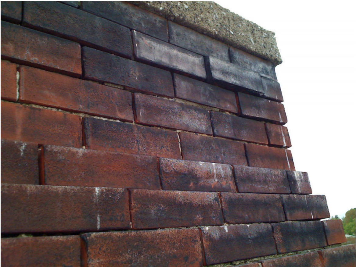
Photo #7: Open brick joints and loose brick at top of chimney
