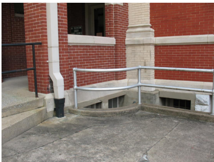
A change in brick at the intersection of the original building (left) and the 1939 addition (right). Also note the deteriorated concrete sidewalk.
