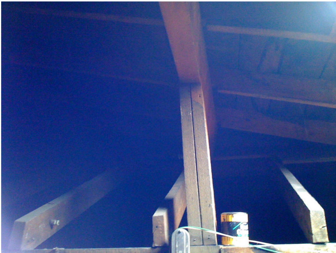
Photo #5: Twisted attic beam rotated away from ends of rafters
