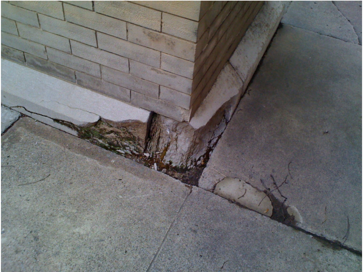
Photo #11: Severe spall at base of exterior masonry column
