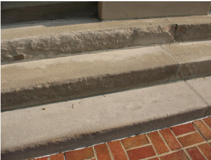
The granolithic steps at the front of the courthouse show signs of deterioration.
