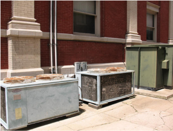
Mechanical units and transformer located on the east side of the building.
