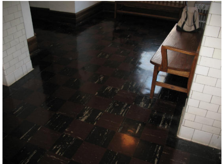
Typical vinyl asbestos tile used in second floor corridor.
