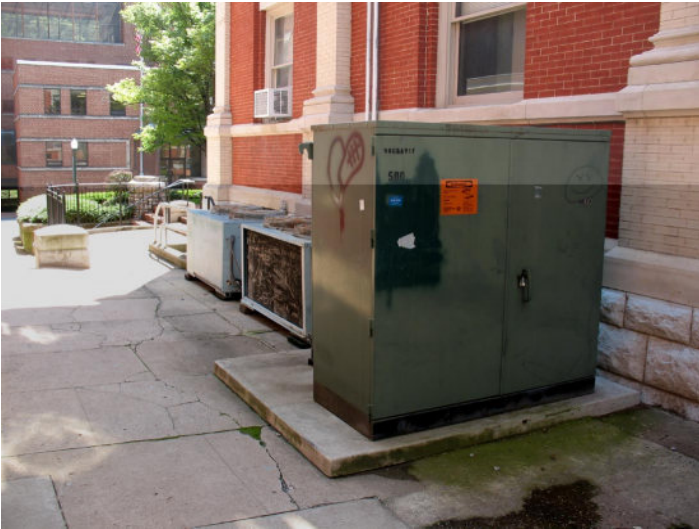
View of transformer and mechanical units on the east side of the building.
