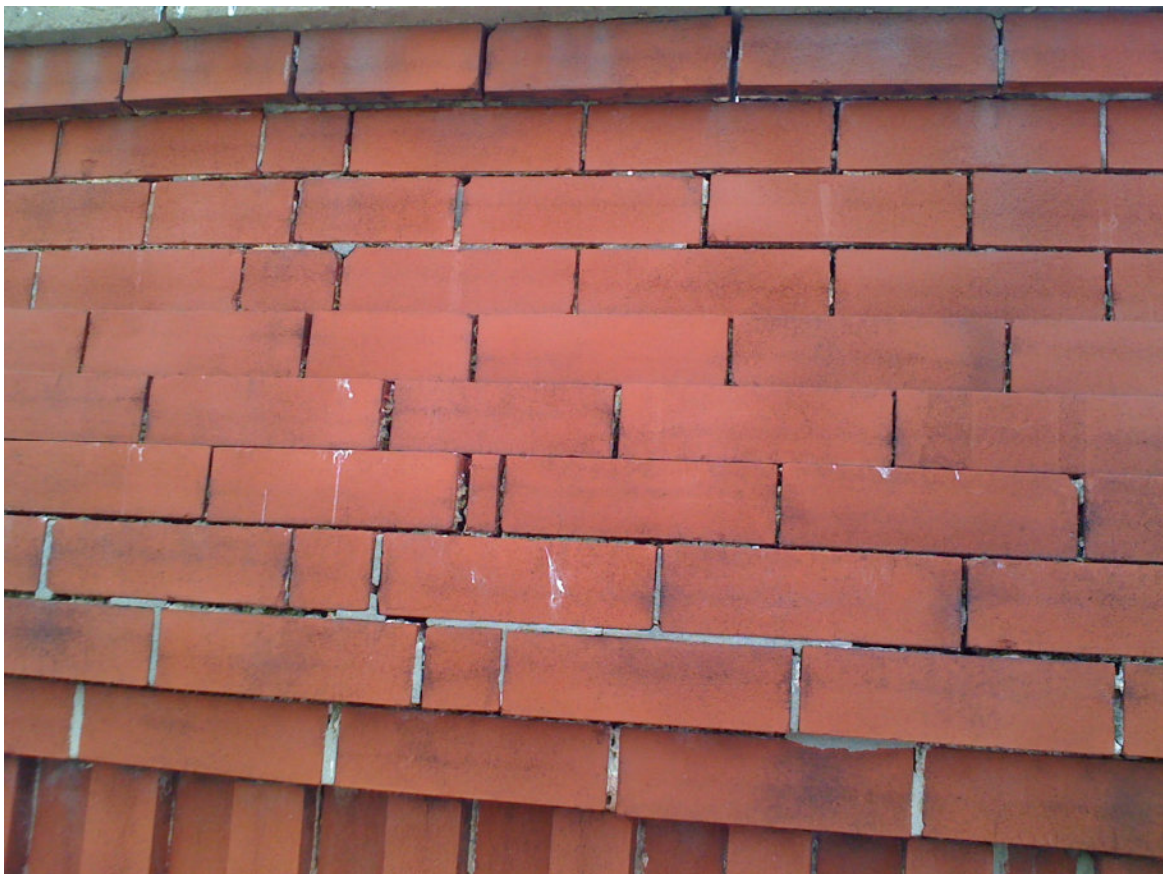
Photo #6: Open mortar joints at top of chimney
