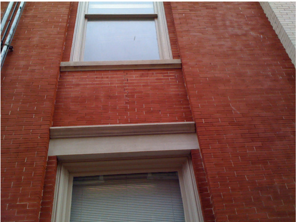
Photo#8: Small vertical crack below 2 nd floor window sill
