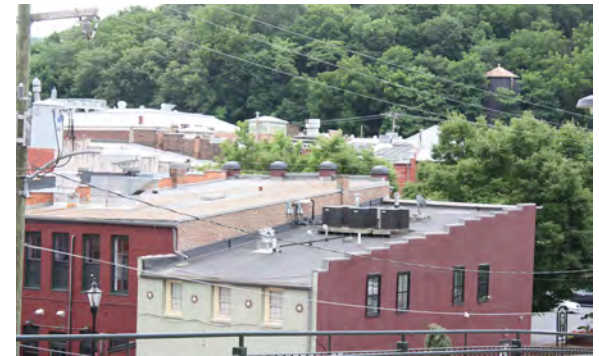
Many of Staunton's commercial buildings' HVAC equipment have roof locations due to the lack of any other open space on the site.
