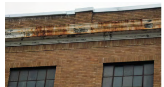
Galvanized metal cornices like this one need a proper primer before painting to avoid rusting.
