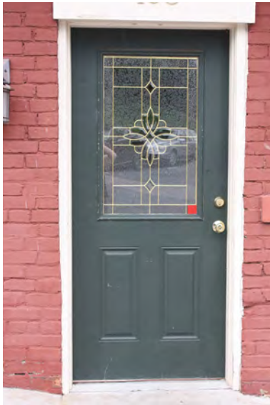
Inappropriate replacement door with artificial stained glass.
