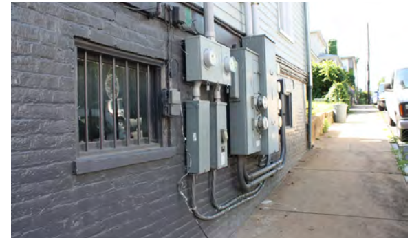
Historic rehabilitation projects should attempt to place utility items on the rear of buildings or other inconspicuous locations instead along a public sidewalk if possible.
