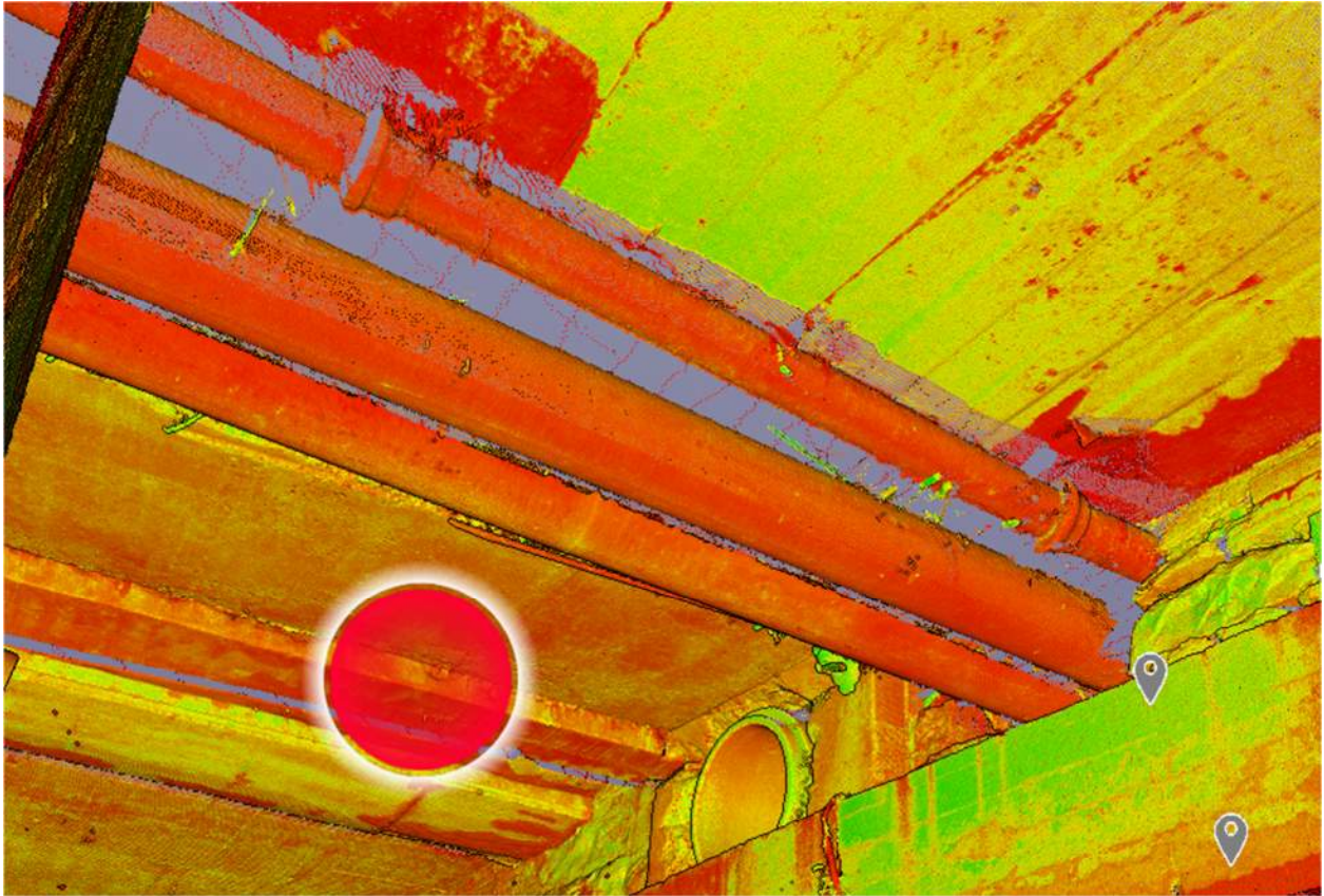
Photo 3 (from TruView Scan) – Gas lines
