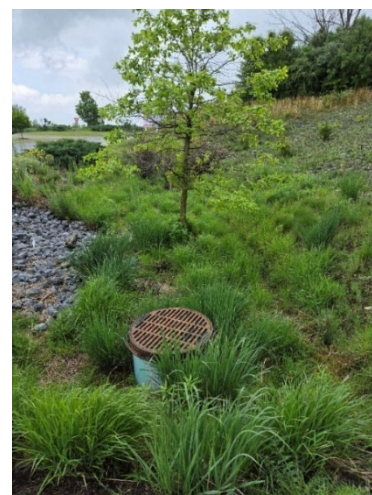
City maintained BMP – bioretention at Crossing Way
