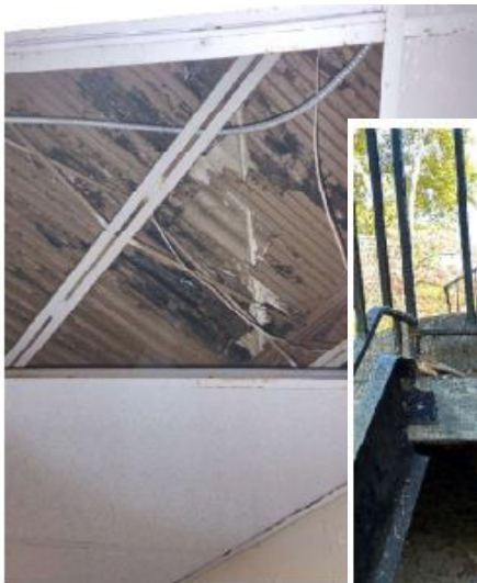
Figure 4 Deterioration of metal deck
