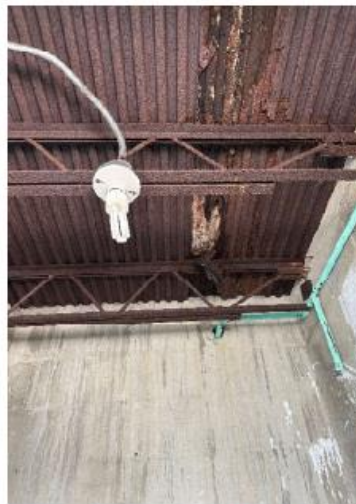
Figure 9 Severely corroded Steel Floor Deck
