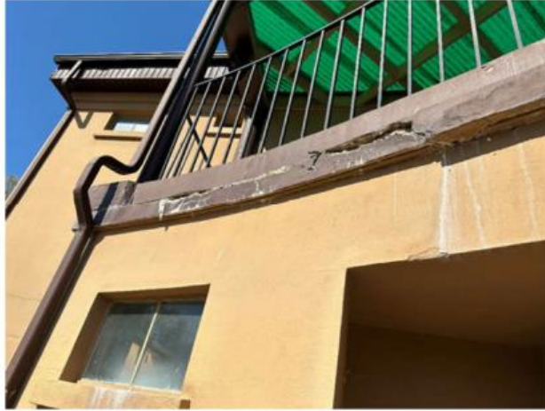
Figure 15 Deteriorated Concrete Slab Edge
