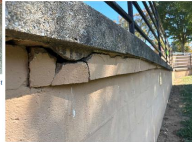
Figure 17 Displaced CMU blocks
