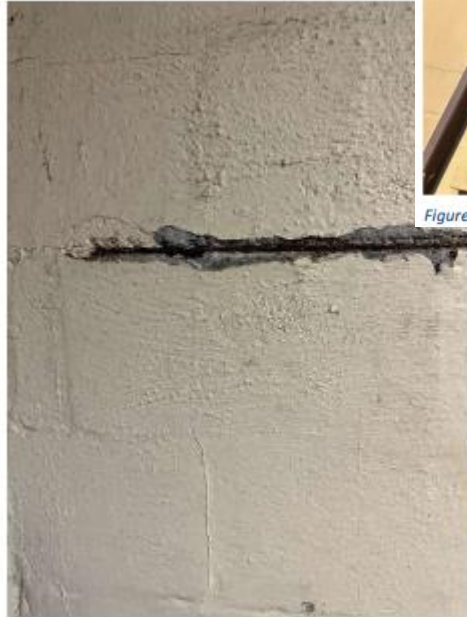
Figure 12 Rusty, Delaminated Horizontal Joint Rebar
