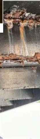
Figure 13 Delaminated, Rusty Steel Tread and Risers of Exterior Stairs to Pool Area
