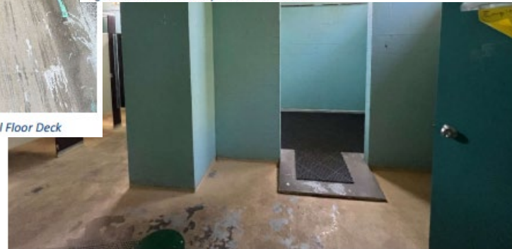
Figure 6 Ramp to shower is not accessible (lip is too tall)
