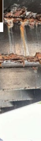
Figure 13 Delaminated, Rusty Steel Tread and Risers of Exterior Stairs to Pool Area
