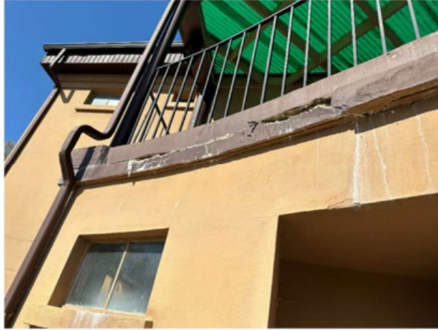
Figure 15 Deteriorated Concrete Slab Edge
