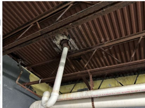
Figure 10 Delaminated Open-Web Steel Joist
