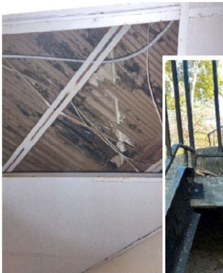
Figure 4 Deterioration of metal deck
