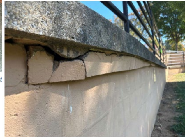
Figure 17 Displaced CMU blocks
