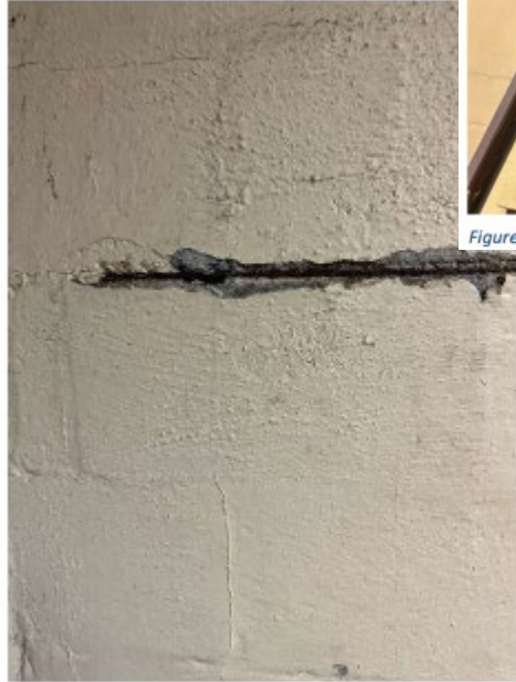
Figure 12 Rusty, Delaminated Horizontal Joint Reinfor
