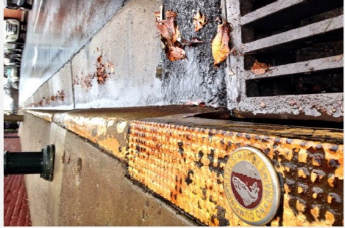
Storm drain in downtown Staunton
