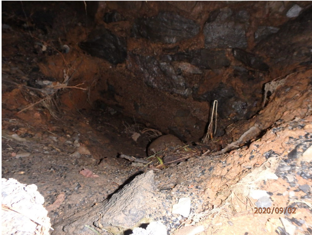
PHOTO 3 - UNDERMINING OF APPROACH PEDESTRIAN PATH AT ABUTMENT B.
