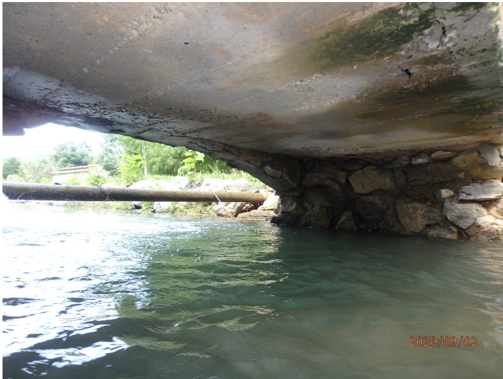
PHOTO 4 - TYPICAL CONDITION OF ABUTMENT AND UNDERSIDE OF DECK SLAB. NOTE SPALLS AND HONEYCOMBING IN DECK SLAB.
