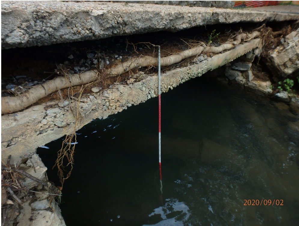
PHOTO 1 - CONDITION OF DOWNSTREAM EDGE OF DECK SLAB AND WEARING SURFACE. NOTE SCOUR (ROD LENGTH = 6'-0").
