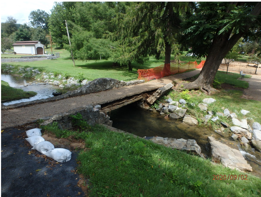
PHOTO 2 - FULL VIEW OF THE DOWNSTREAM FACE OF THE STRUCTURE. NOTE FAILED WINGWALL AND DECK FAÇADE AND AREA OF LIGHT EROSION.
