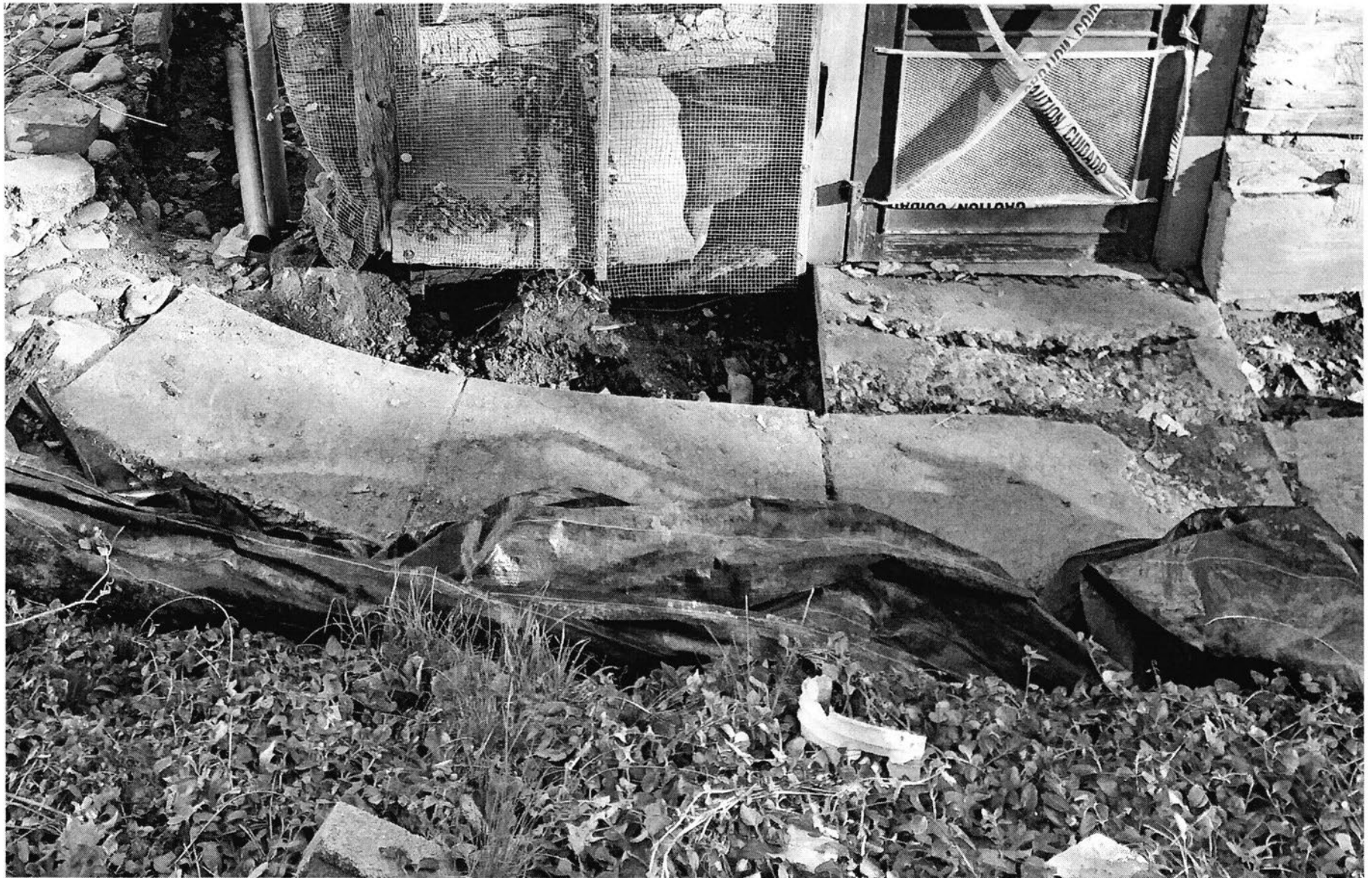
Entry Walk - view from East Beverley Street. Eroded/broken surface at door. Walk extends from concrete steps. Made of modern, gray concrete with no discernible fine aggregate. #57 stone aggregate under surface layer. Estimated date of construction is post 1987.
