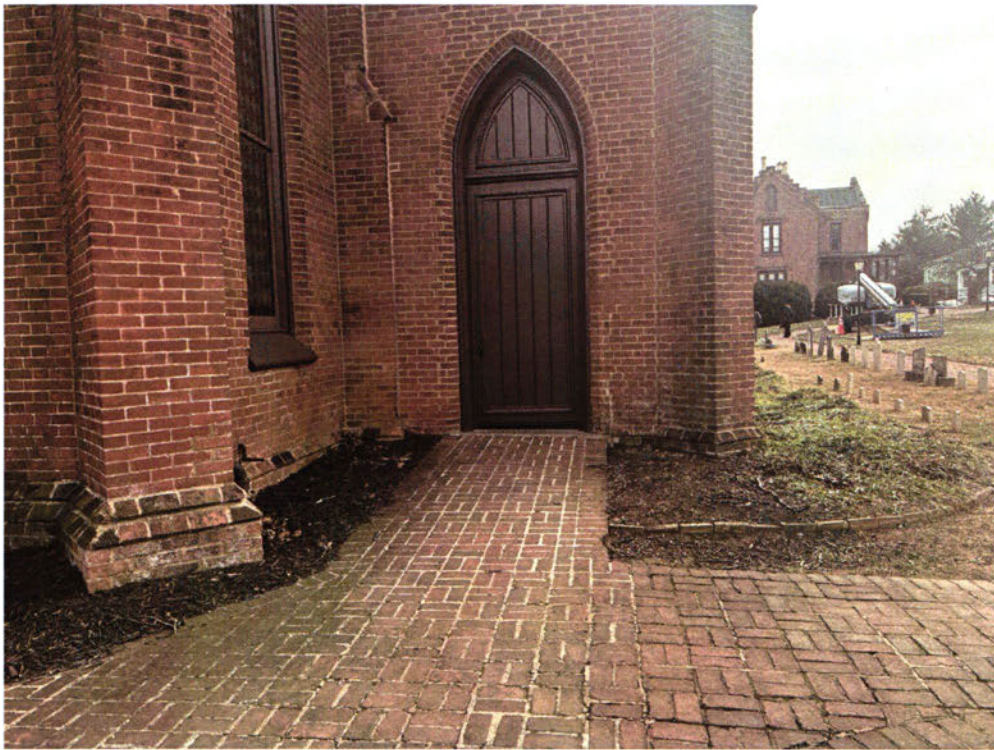
Trinity Church's only handicapped accessible doorway.
